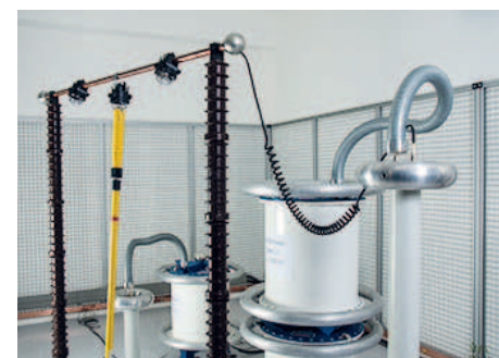
High voltage laboratory
